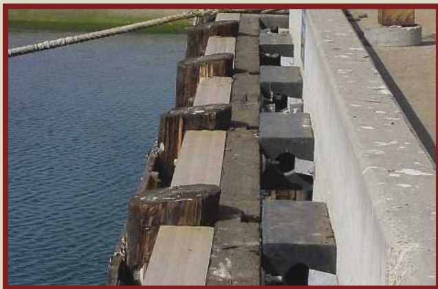
Figure 1a. — Examples of prototype WPC products from Washington State University’s Wood Materials and Engineering Lab. From top: extruded sill plate; chock members being drilled for installation at Port Hueneme, California; installed chock members.
